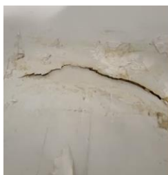
Tub whit crack repair on bottom
