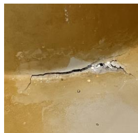
Shower stall whit crack
